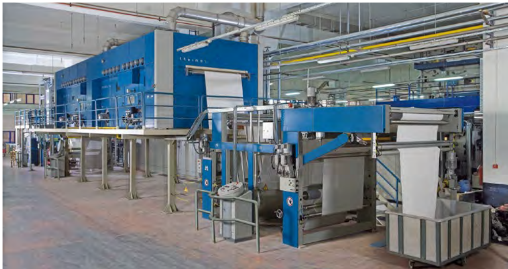
A recent Thermex installation in Italy © 2023 Monforts
